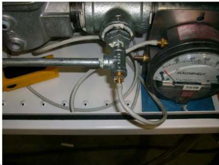
Test Port at Tee for Pilot Tube
